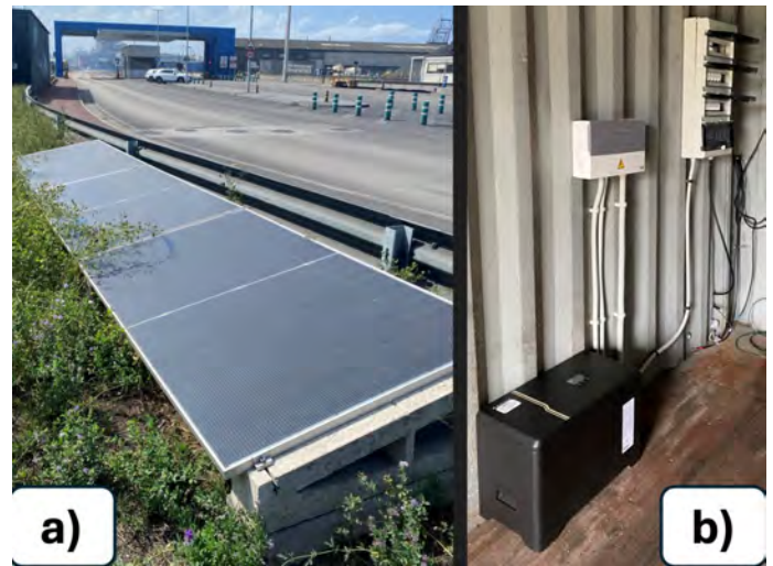
FIGURE 3: a) Solar panels on support structure and b) Solar equipment control system and storage battery.
